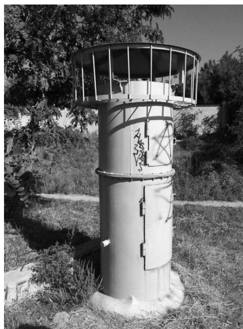
Fig. 2. Current plants of dry chemical filtration among park areas
