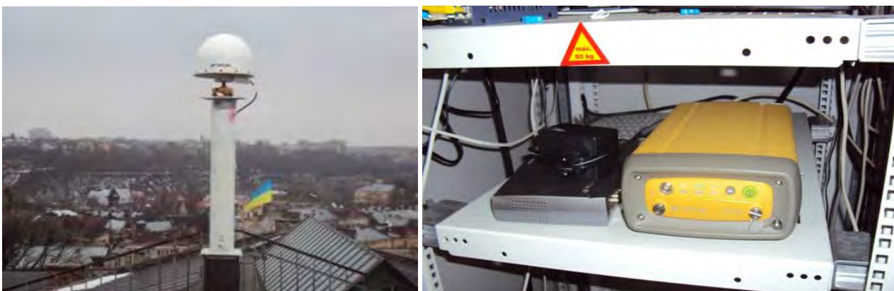
Fig. 1. GNSS equipment of the SULP station
