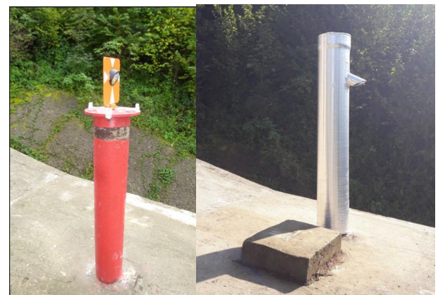
Fig. 5. Reflector with special thermal protection fixed on the anchor pillar
