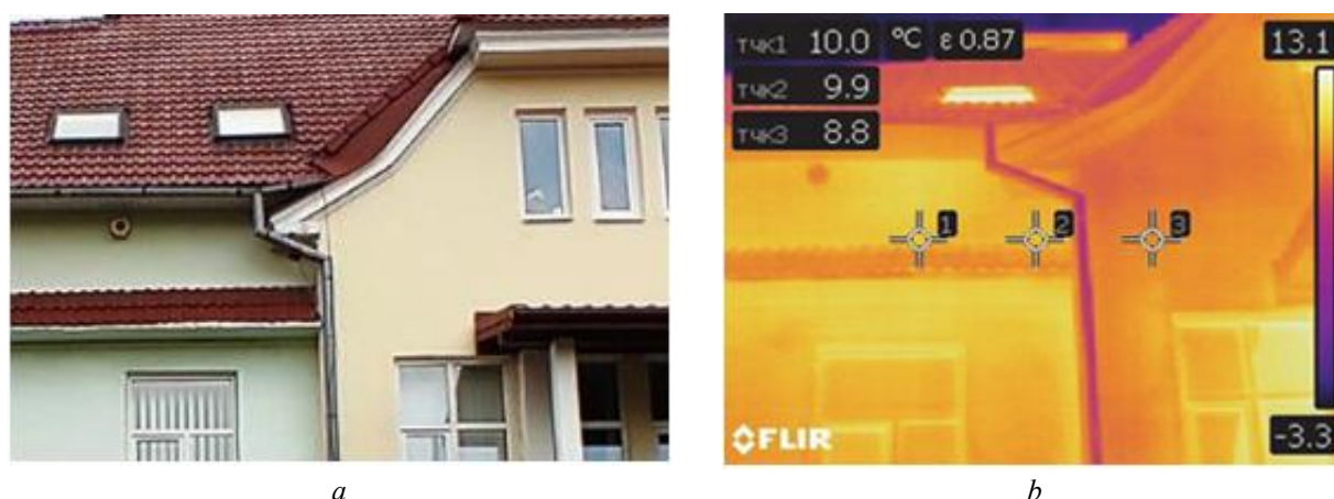
Fig. 2. Results of thermal imaging of an element of the external facade of the building. a) photo of the element of the facade of the building; b) temperature field of the facade element
