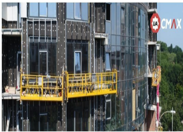
Fig. 2 Installation of glass blocks and elements for the realization of modern buildings
