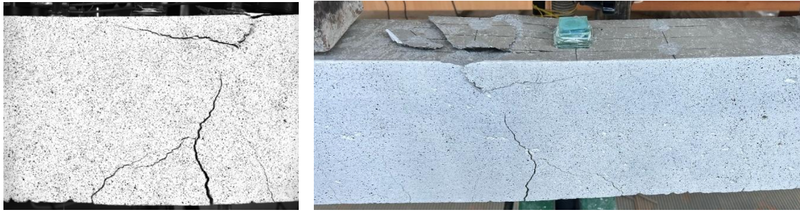
Fig. 9. Appearance of cracks during the failure of the restored RC beam.
