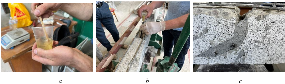
Fig. 8. Crack injection process: a – mixing the epoxy resin; b – injecting epoxy resin into the crack; c – sealing the packers and completing the crack injection.
