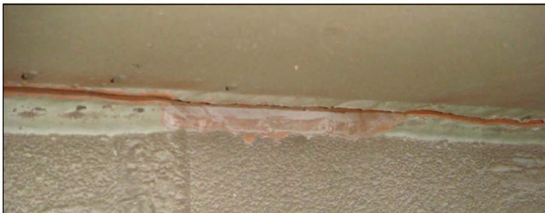
Fig. 1. Typical fatigue cracks in the web-flange connection area of steel runway beams
