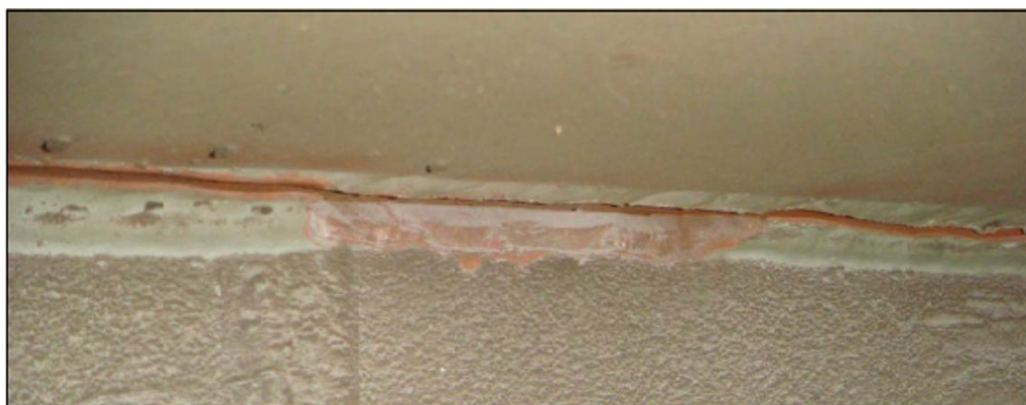
Fig. 1. Typical fatigue cracks in the web-flange connection area of steel runway beams
